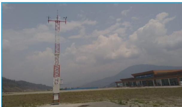
CWIS installed at Pakyong Airport, Sikkim
