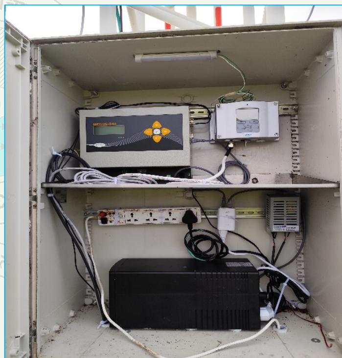
DCWIS (at RWY 05) and PWD (RWY 23) Systems installed at Rajahmundry airport
