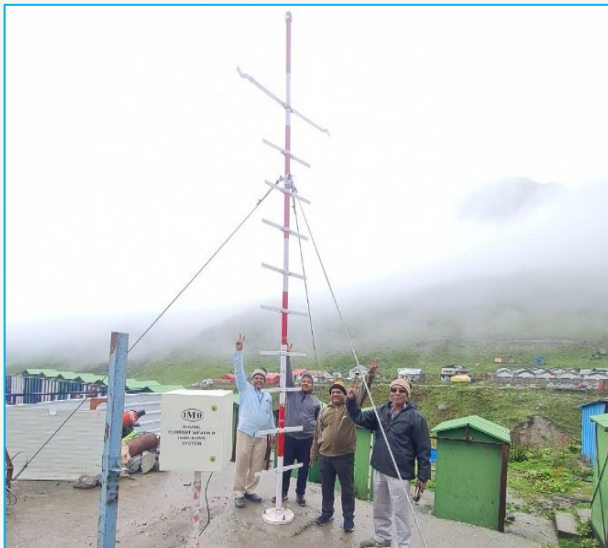
H-AWOS installation at Kedarnath ji
