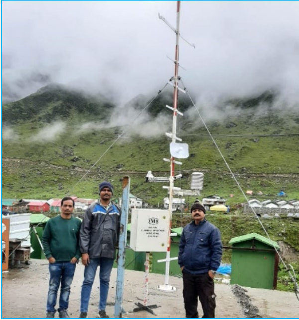
H-AWOS installation at Kedarnath ji
