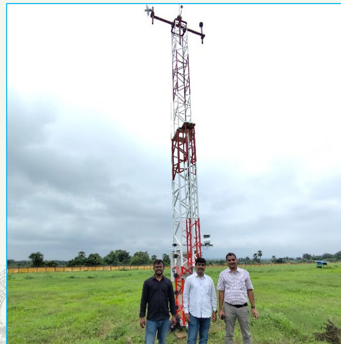
DCWIS (at RWY 05) and PWD (RWY 23) Systems installed at Rajahmundry airport
