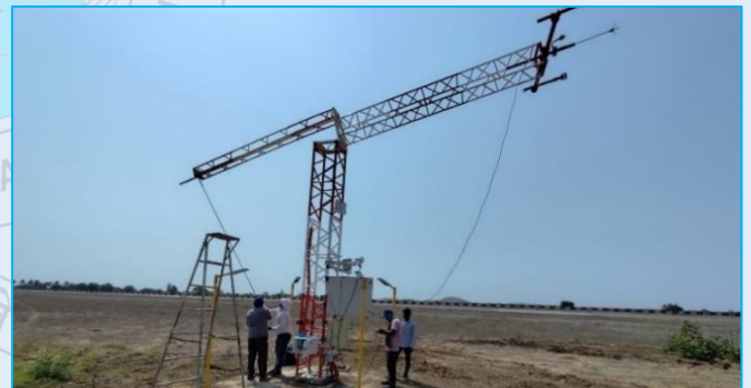
DCWIS & PWD at Keshod Airport
