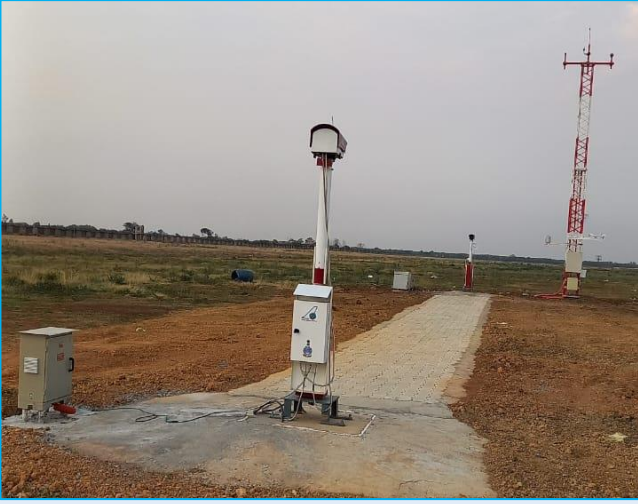
Drishti Transmissometer at Raipur Airport
