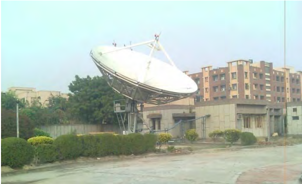
VSAT Hub Antenna (9.0 m) at NCMRWF Complex, Noida
