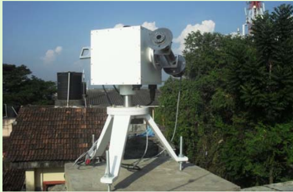
Pyrhelimeter on Solar Tracker V-SOL-2A2P at, Goa
