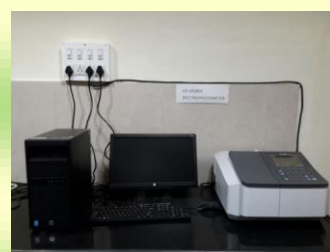
Fig. 16. Ion-chromatograph, UV-VIS Spectrophotometer and Semi-micro Balance installed in Air Pollution Laboratory, Pune
