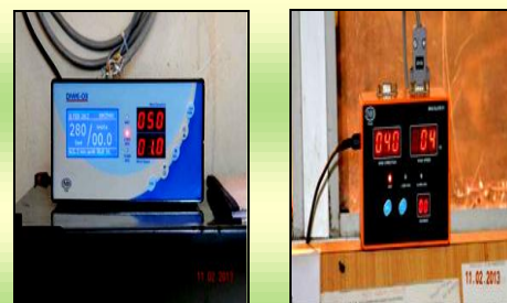
Fig. 13. DIWE System on touchdown zone of runway, DIWE Data Logger and DIWE Display Unit
