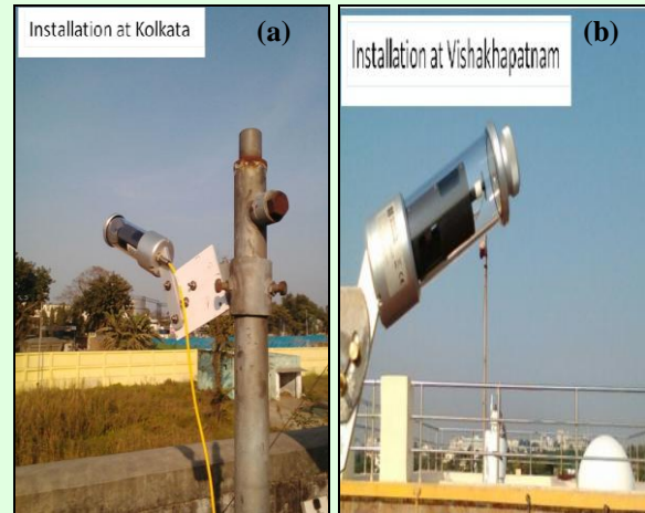
Fig. 6(a&b). Installation of electronic sunshine recorder at (a) Kolkata (b) Vishakhapatnam
