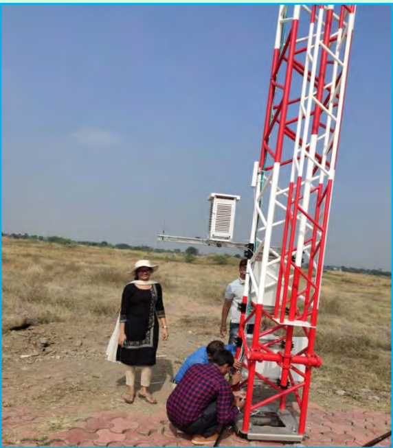
Fig. 17. DCWIS System installed at Shirdi Airports
