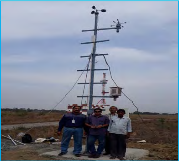
Fig. 16. DCWIS System installed at Gaya Airports
