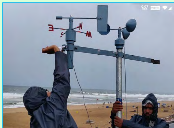
Fig. 11. HWSR installed at Puri
