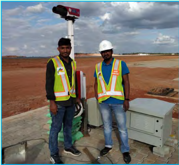
Fig. 12. Drishti Transmissometer systems installed at Bangalore (new runway) airport
