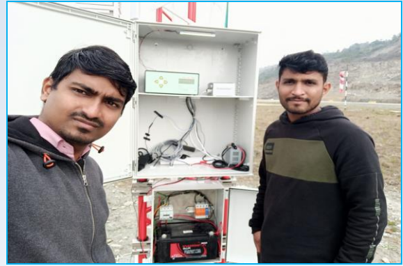
Fig. 9. DCWIS system installed at Pakyong
