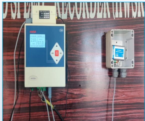
Fig. 10. HWSR installed at Vishakapatnam
